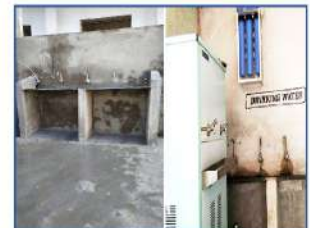
Ro Plant & Water Cooler
