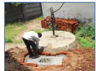
Rainwater Harvesting System
