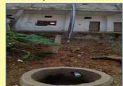
Rainwater Harvesting System
