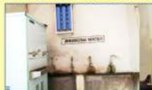
Ro Plant & Water Cooler
