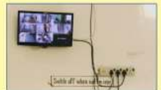
24Hrs. Cctv Vigilance
