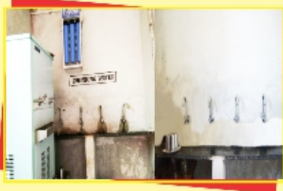
RO PLANT & WATER COOLER
