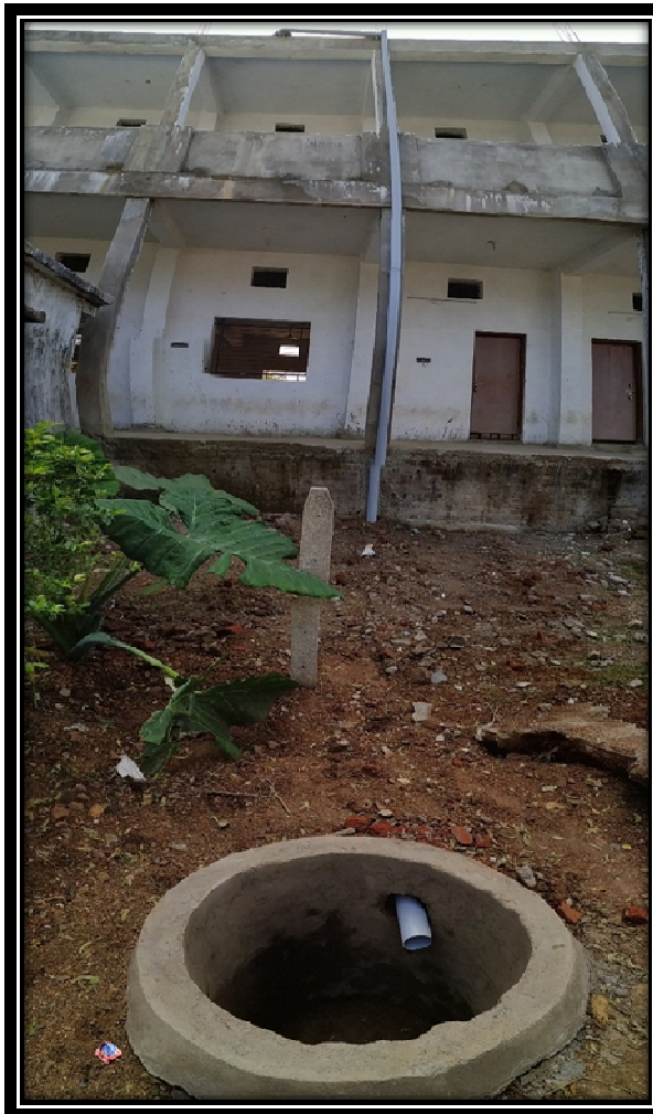
Rainwater harvesting system
