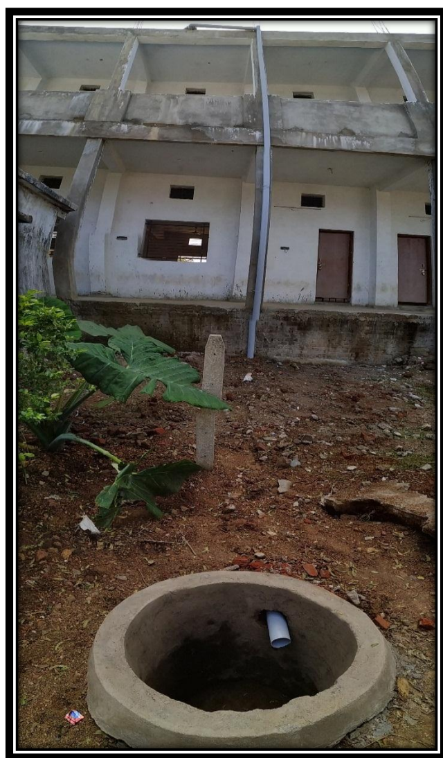
Rainwater harvesting system
