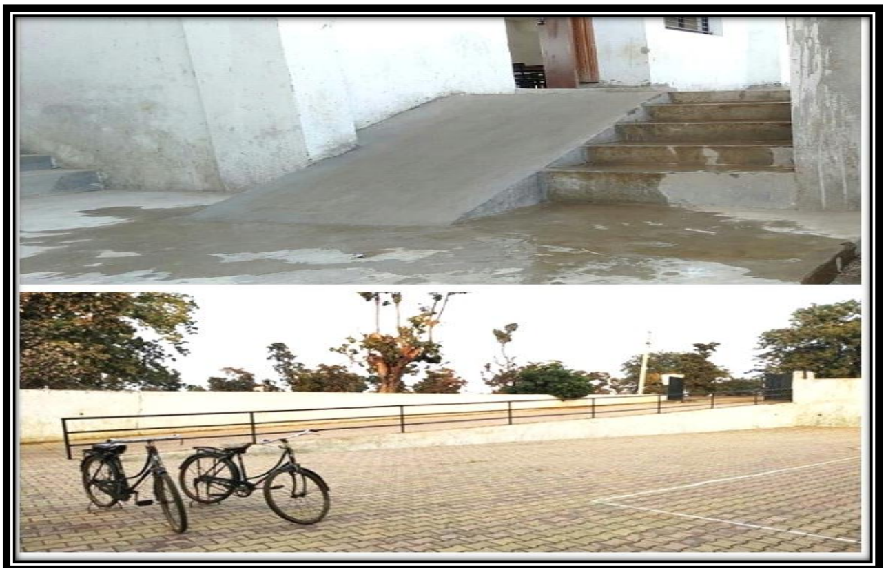
Ramp facility for person with disability
